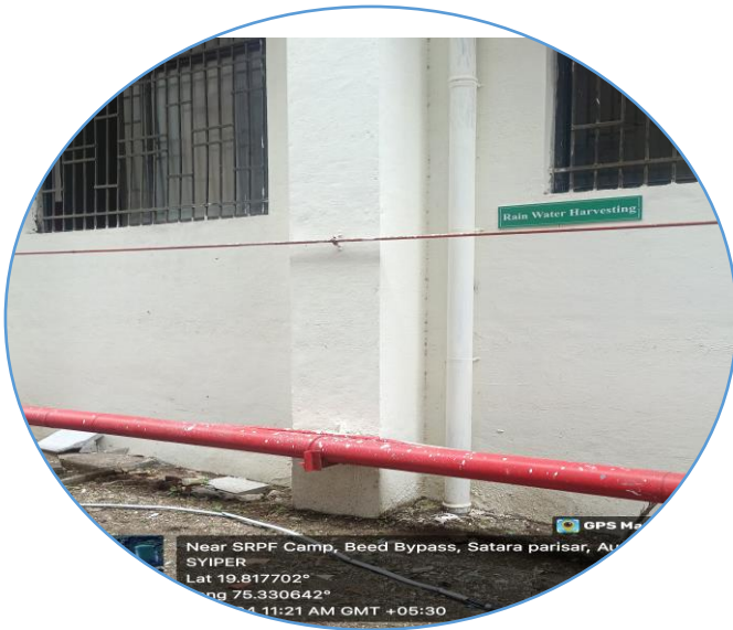
RAIN WATER HARVESTING SYSTEM
